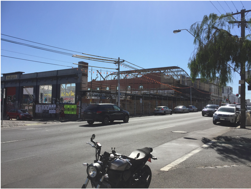
View across Johnston St to 239-247 Johnston Street, Fitzroy During demolition. (Former Lyric Theatre, Now Aldi)
